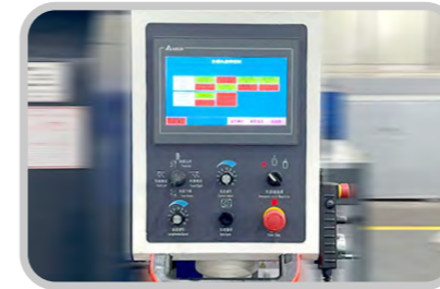
Omron PLC with touch screen
