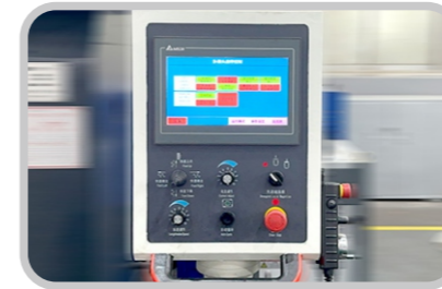
Omron PLC with touch screen
